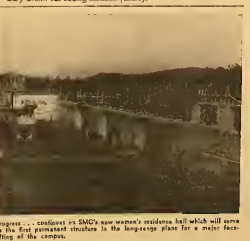
Progress . . . continues on SMC's new women's residence hall which will come as the first permanent structure in the long-range plan for a major facilities of the campus.
