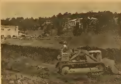
Excavation . . . Makes way for foundation of the new women's residence hall, which will house 320 women.
