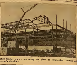
Steel Girders . . . are swung into place as construction contract is won by SMC.
