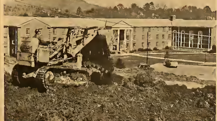
As the new administrative building moves toward the hoped-for completion date of Christmas '66, this bulldozer prepares site and furnishes alternative noise to teachers' lectures in Lynn Wood Hall.
