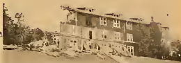
Old Talge Hall loses part of its south wing as wrecking crews knock it down. The porches fall down as demolition started.
