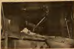
Last coal-fueled boiler was removed from "soot factory" on SMC campus in October.
