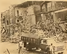
Getting rid of the debris was as much of a problem as tearing down the building. Most of it was moved out and burned, since there was little salvageable.
