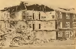
Room partitions, halls, and doors are revealed in giant cross section of the back of the building.
