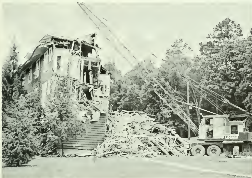
Wrecking crew brings down the north wing of old Talge Hall to make way for new library.
