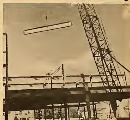
Construction on the new library is progressing rapidly, as can be seen from this picture of the steel workers in action. (Photo by Adams)
