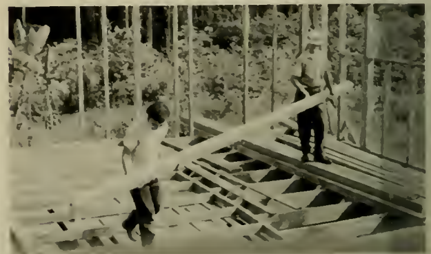
Gladstone Simmons, junior theology major, takes time from pastoring to build on the house. Hard-hatted Ray Wagner from North Carolina directs construction of the house.
