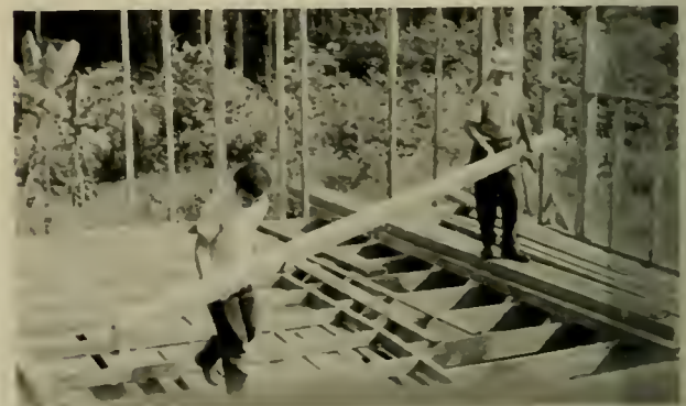
Gladstone Simmons, junior theology major, takes time from pastoring to build on the house. Hard-hatted Ray Wagner from North Carolina directs construction of the house.
