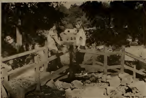
Roy Armstrong &amp; Julie Jacobs enjoy the scenery at the "Alcove" which is presently under construction.
