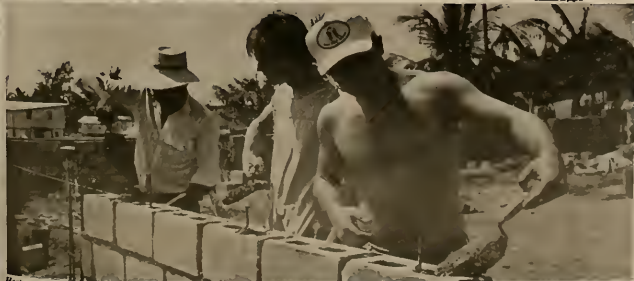
Hector, a local Hondurian, Dravis Golightly, and Steve Kriener fill a wall with cement. The wall is part of a new market-place for the villagers in Honduras. (See story on page 4.)
