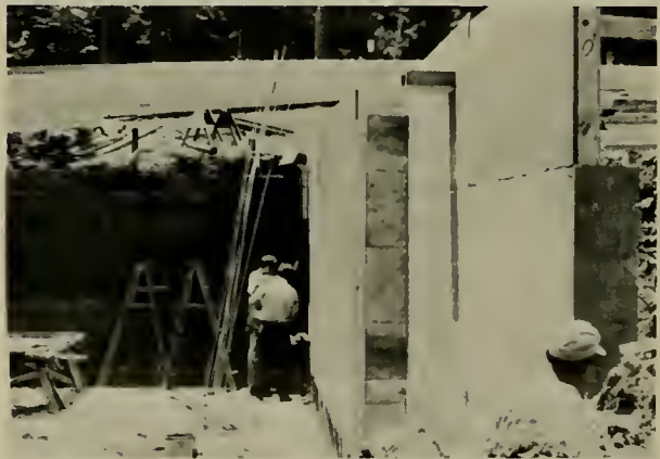
Foundation goes in for new building being financed by SMC's Committee of 100.
