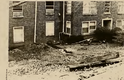
What a Mess! The digging that has been taking place around campus is for fiber optic cables that will be used to upgrade the communications system. Talge Hall, above, is one of the buildings that will benefit from the new cables.
