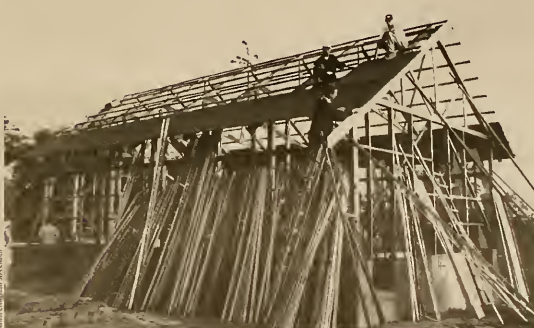
Christmas in Cambodia: During the Christmas vocation of '96, 30 members of the Collegedale SDA Church traveled to Cambodia to build this church (above) for a local SDA congregation.
