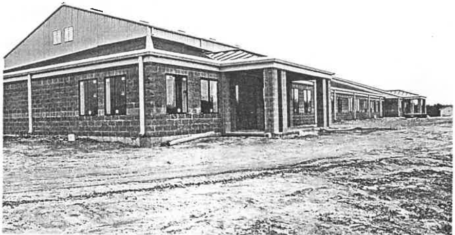
The 22,355 square foot multipurpose building contains a gymnasium, cafeteria, classrooms, administration offices, and will temporarily house the bakery.
