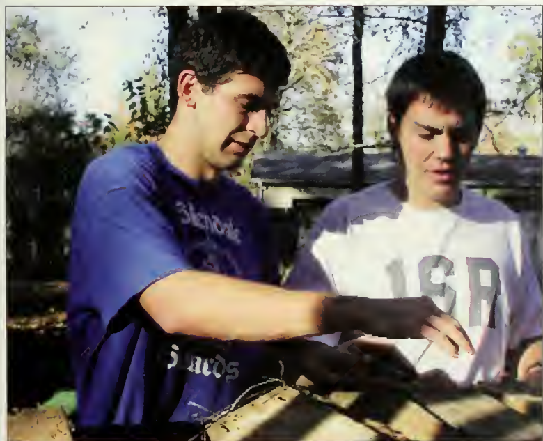
A mini-grant from American Humanics helped Grunt Ministries reconstruct a local family's dilapidated porch. Jonathan Fetrick and Stephen Lundquist sort beams.
