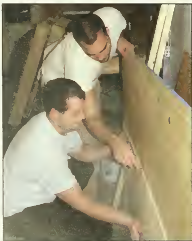
Students build shelving to transform a cargo trailer into a mobile outdoor school.
