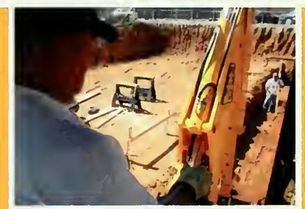
Construction begins on a building that will bring a new level of excellence to wellness on campus.
